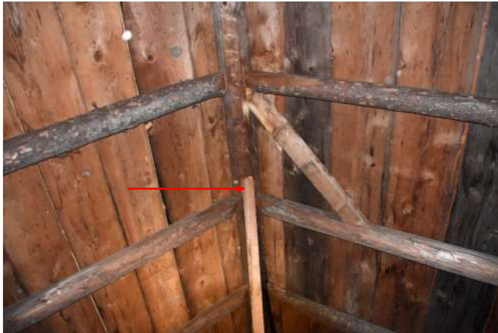
Figure 3, Separation of Diagonal Brace and Ridge Beam
