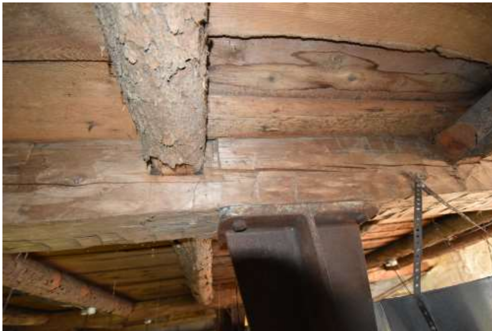
Figure 5, Splitting of Beam near Mortise and Tenons Joint above Truss Post
